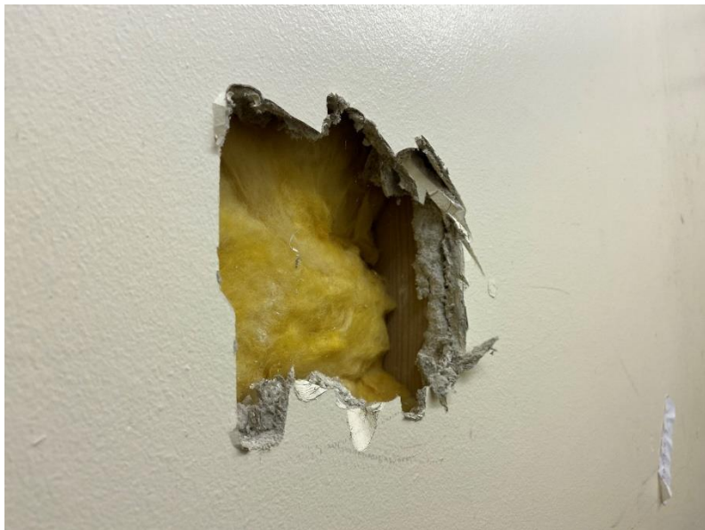
Figure C.3: Hole in partition between Music Practice 15 and Circulation 13
