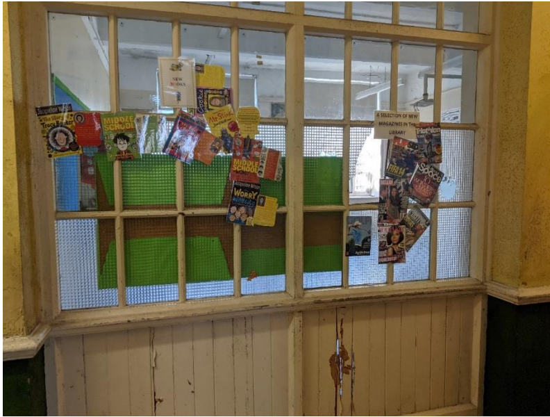
Figure C.2: Glazing smashed of Classroom 26
