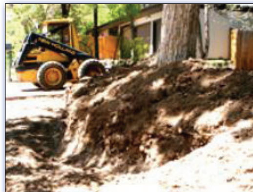
Photo 8 Examples of poor excavation activities.
