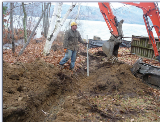
Photo 7 Examples of poor excavation activities.
