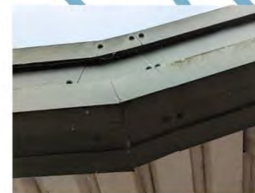
Figure 21 - Gaps under metal fascias and soffits.
