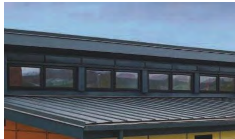
Roof to Extension - metal standing seam roof colour Matt RAL 9007 Orion Grey
