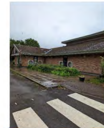
Figure 19 - Western aspect of the building (area of roof to be affected by the works).
