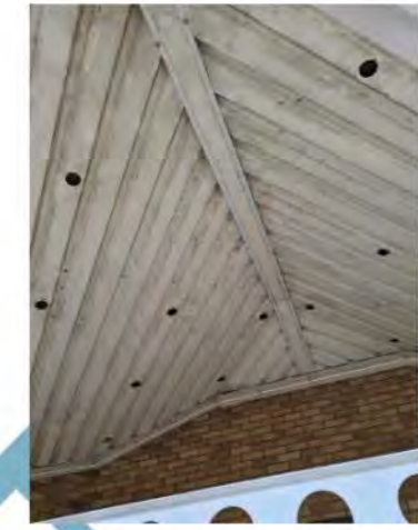
Figure 18 - Ventilation holes under the roof at the main entrance to the building.
