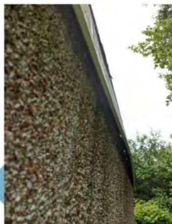
Figure 24 – Gaps between flat roof and wall of the nursery.
