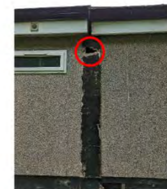
Figure 22 - Gap between the nursery building.
